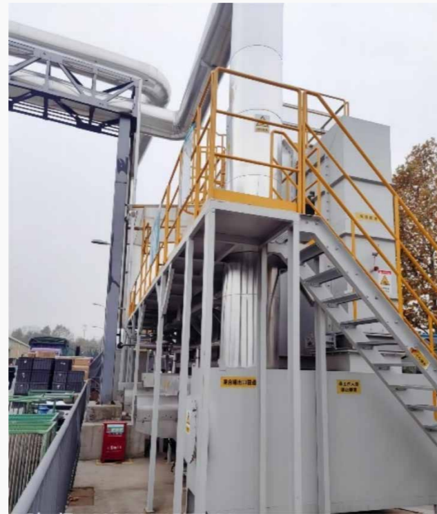
Qingdao Hisense Hitachi Air Conditioning VOCs Exhaust Gas Emission Treatment Demonstration Project
